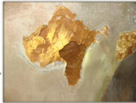
Tunnel lining damage in the east infiltration gallery
