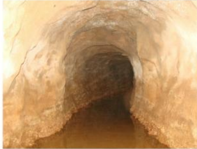
West Infiltration Galleries ~270ft
